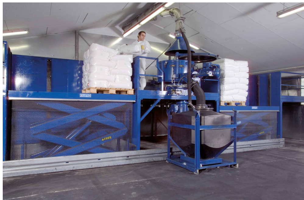
Eco-friendly and on the cutting edge of technology: carbon black mixing area in compliance with ATEX guidelines under directive 2014/34/EU
